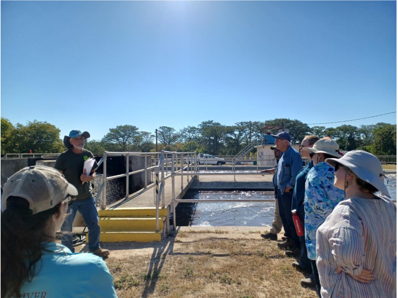
Participants of the grassroots gathering of water advocates on a tour of the Bandera wastewater treatment plant, led by plant manager John Heggemeier (left). Photo courtesy of the Hill Country Alliance.
