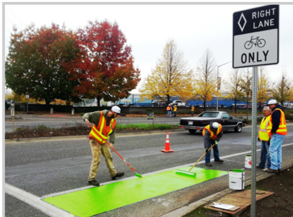
WORKERS PAINTING A BIKE LANE BRIGHT GREEN. PHOTO SOURCE: SEATTLE DEPARTMENT OF TRANSPORTATION
