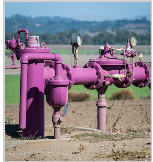
Purple pipes are used to indicate water is not potable or drinkable. (CC) FLICKR
