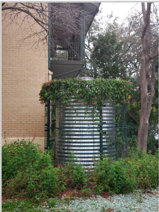
RAINWATER HARVESTING SYSTEM PHOTO COURTESY HALFF ASSOCIATES
