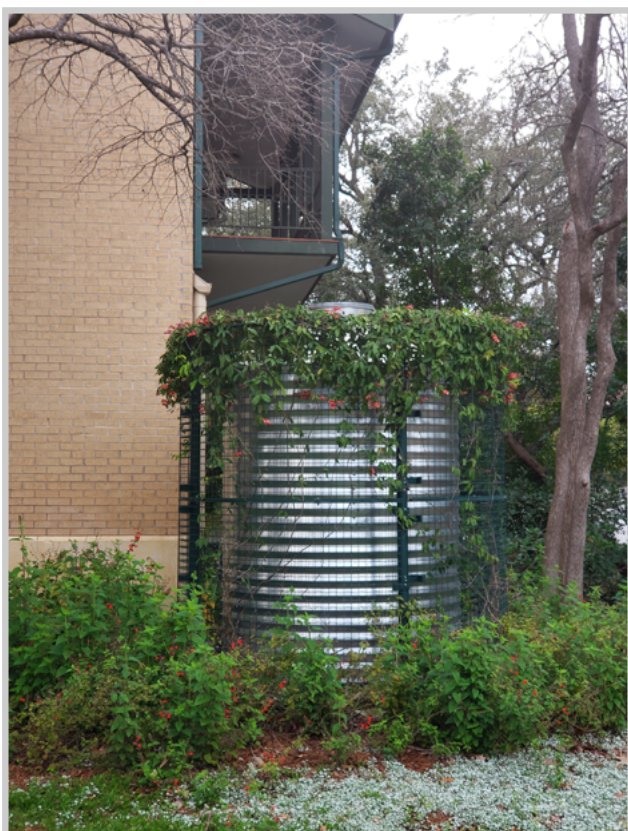
RAINWATER HARVESTING SYSTEM PHOTO COURTESY HALFF ASSOCIATES
